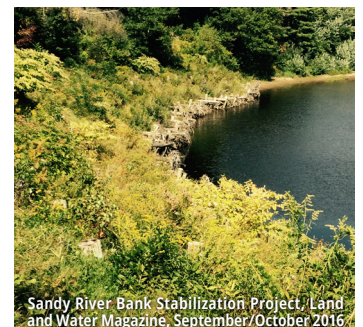
As a result of Hurricane Irene in 2011, followed by an intense rain event a week later, a highly accelerated river flow undermined and collapsed this 50-foot section of the riverbank in Farmington Falls, affecting Whittier Road, an important thoroughfare. Root wads were installed as a mitigation measure for deflection of flow energy away from the badly eroded outside bend, and to provide fish and animal habitat. The slope was planted with a variety of seedlings.
