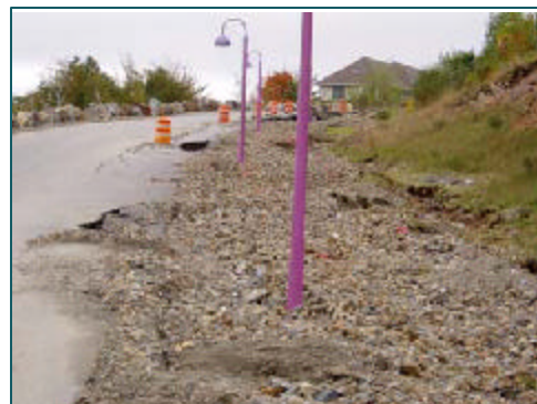
Degraded road at Birch Bay Village
